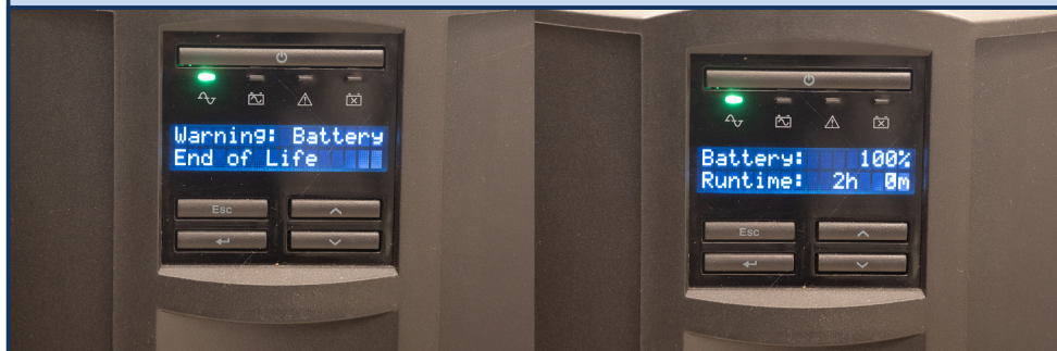
Fig. 1: Contradictory indications on the UPS
